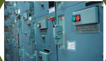
Industrial Control Panels
